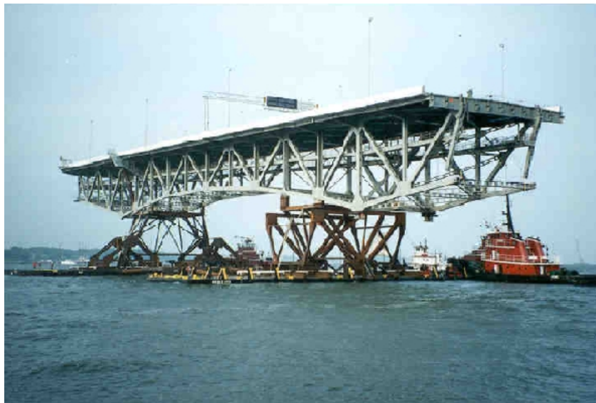
Figure 5.4: Truss PCU being barged in for the George P. Coleman Bridge (FHWA 2004)
