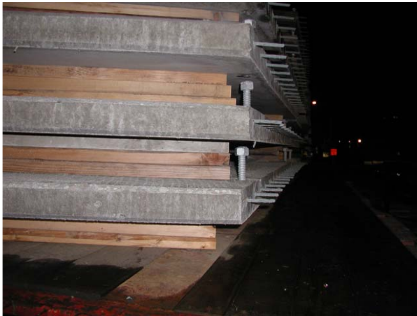
Figure 3.8: Panels stacked on site with leveling bolts and prestressing extensions visible (Courtesy of WSDOT)
