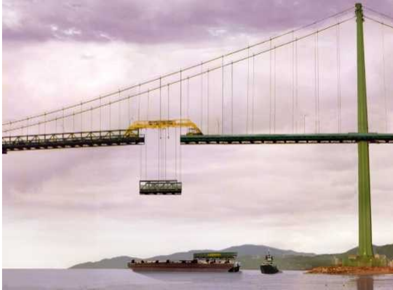
Figure 5.5: PCU being raised into place on the Lions' Gate Suspension Bridge, Vancouver, B.C. (FHWA 2004)
