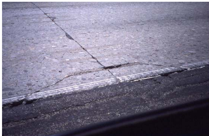
Photo 5. Corner cracking resulting from traffic loading when sawcuts penetrate too deep in the concrete roadway.
