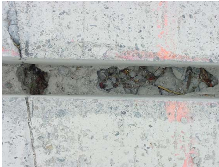
Photo 37. Patching material was poorly consolidated beneath the dowel bar, which may result in pop out of patching material.
