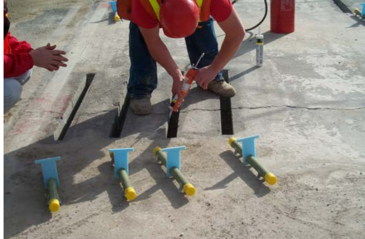
Photo 18. Caulking should be placed along the sides and bottom of the slots.
