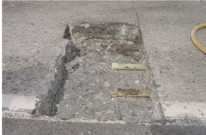
Photo 26. Epoxy coated dowel bars that have corroded possibly due to improper handling.
