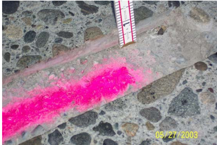
Photo 36. Patching material placed too low, results in poor ride quality and may cause cracking due to insufficient cover on bar.
