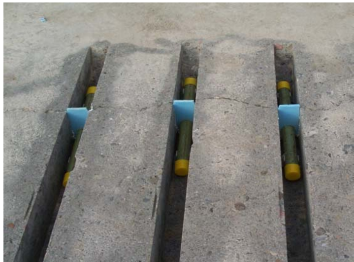
Photo 22. Dowel bars that have been placed and aligned in slots over a transverse crack.
