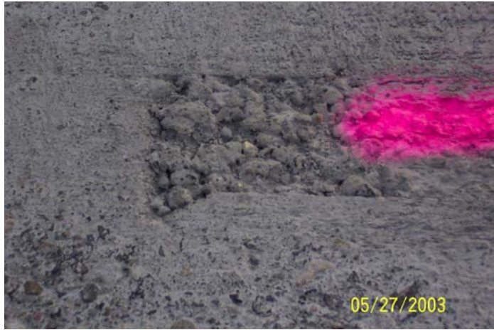
Photo 35. Segregated patching material, which may lead to additional spalling and cracking.
