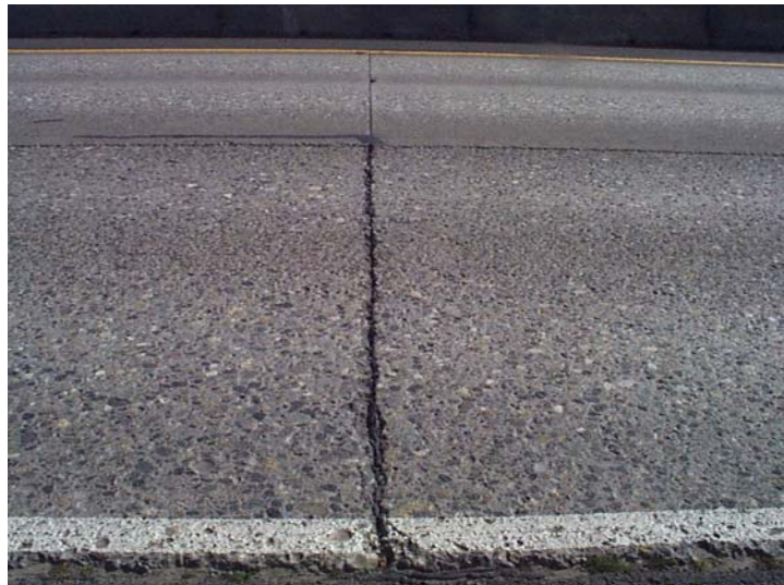
Photo 40. Rotomilled surface. The transverse joint has been damaged due to the impact of the rotomill on the concrete.
