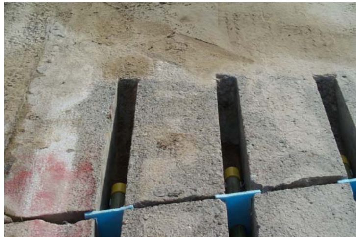
Photo 17. Sandblasting debris adjacent to slots should be cleared to avoid contamination during placement of patching material.
