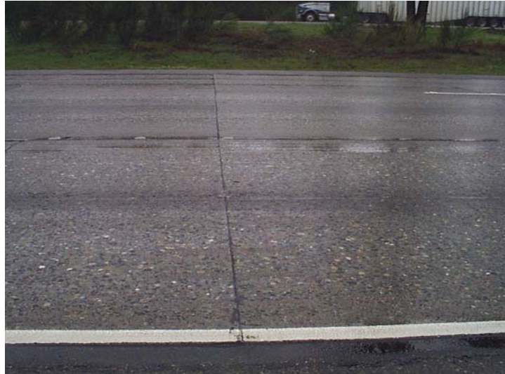
Photo 39. Diamond ground surface. The transverse crack has not been damaged.
