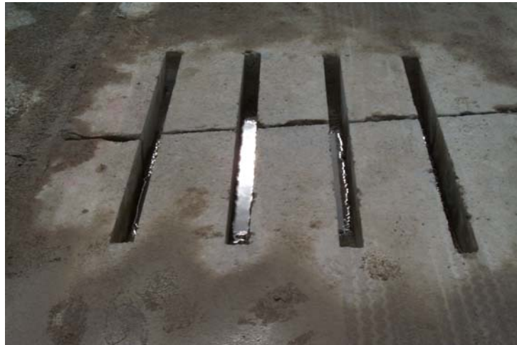
Photo 16. Removal of water, from slots, is required prior to placement of patching material.
