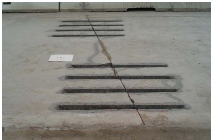
Photo 3. Dowel bar retrofit slots placed parallel to centerline over a skewed joint.
