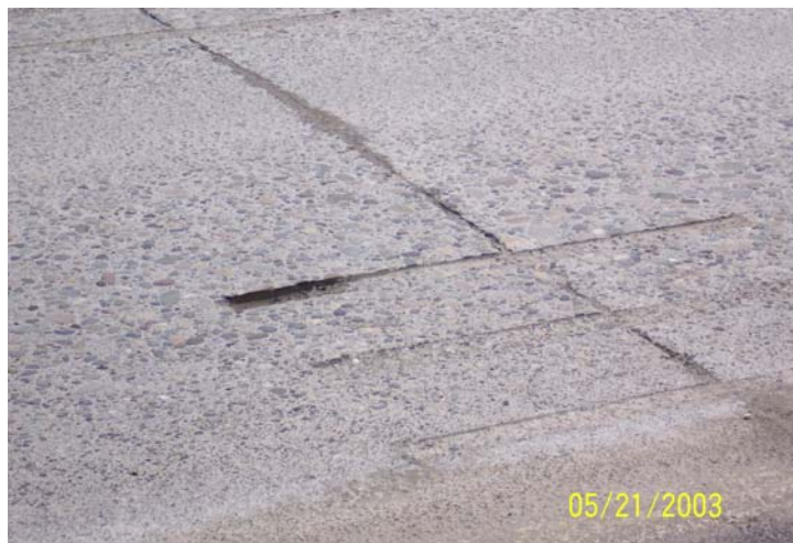
Photo 38. Opening to traffic prior to proper curing of patching material.
