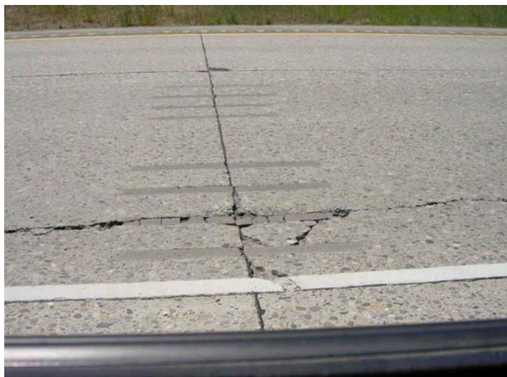
Photo 6. Existing longitudinal crack that intersected a dowel bar retrofit slot.
