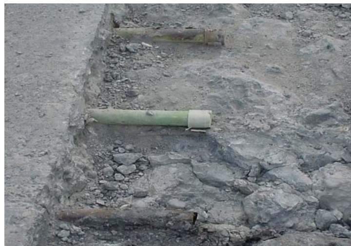
Photo 25. Epoxy coated dowel bars that had chips and nicks prior to placement. The corrosion, which resulted two years after placement, could have resulted from improper handling.
