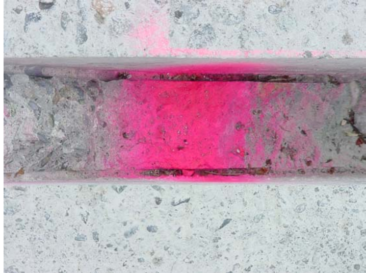
Photo 10. Concrete improperly removed from the bottom of the slot.
