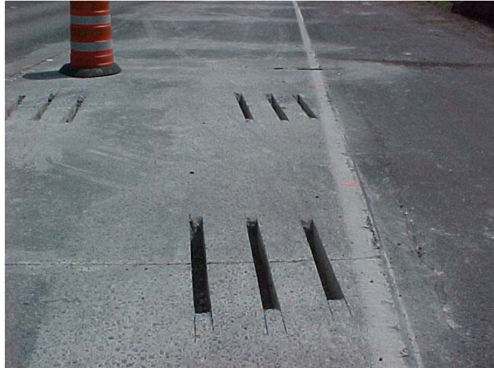
Photo 4. Slots should not be placed perpendicular to skewed joints.
