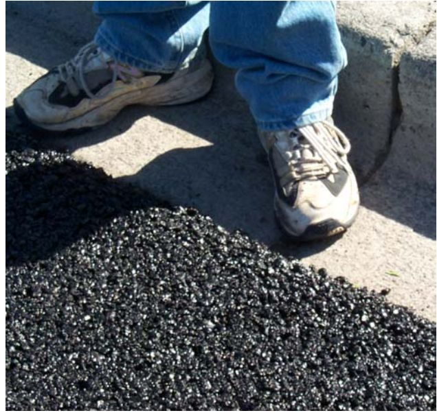
Photo 12. NovaChip® asphalt placed adjacent to curb and gutter. Rotomilling adjacent to the curbing was not done. Previous surfacings and the NovaChip® left a trough in the gutter.
