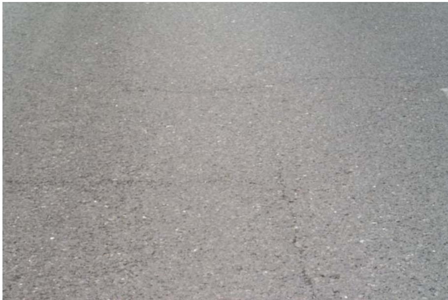
Photo 28. Block Cracking reflecting through the NovaChip ® overlay.
