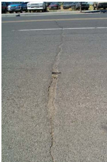
Photo 5. Medium to high severity transverse crack seen on SR 17. Cracks of this width should be crack sealed prior to overlay.
