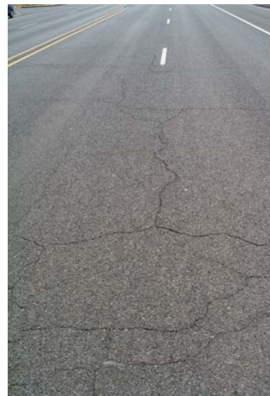
Photo 6. Cracks less than ¼ inch observed in Soap Lake. Crack sealing or repair is not necessary.
