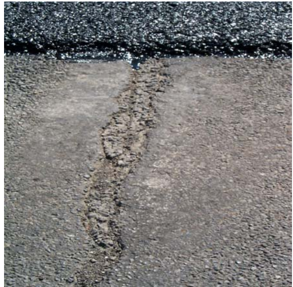
Photo 10. NovaChip® asphalt placed over existing cracks. These transverse cracks should have been sealed prior to the NovaChip®.
