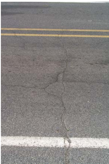
Photo 4. Typical transverse crack observed on SR 17 in Soap Lake. Repair or crack sealing is not necessary for cracks ¼ inch and less.
