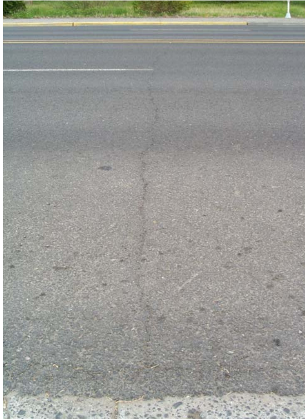
Photo 27. Transverse crack reflecting through the NovaChip ® overlay.
