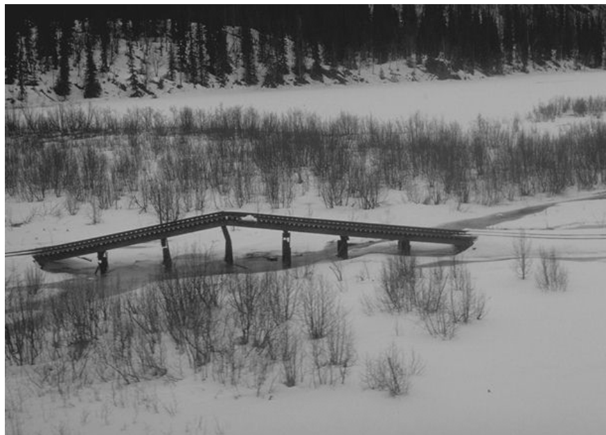
Figure 3.2. Buckled railroad bridge between Portage Junction and Seward, Alaska. A total of 92 highway bridges were severely damaged or destroyed, and 75 railway bridges were moderately to severely damaged (McCulloch and Bonilla, 1970).
