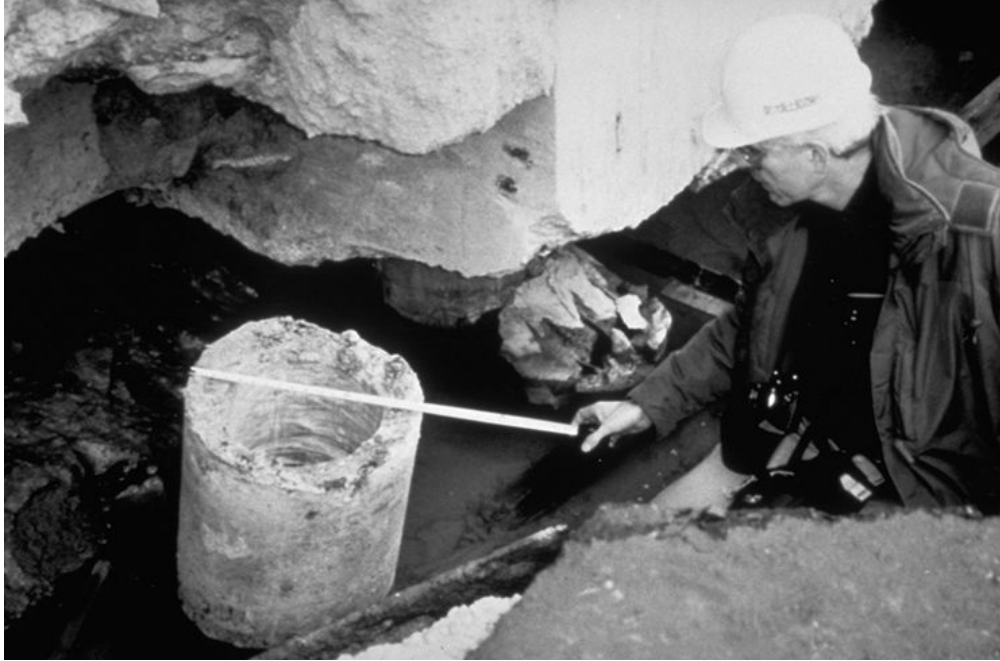
Figure 3.3. Damage to pile foundation in 1995 Hyogo-ken Nambu earthquake.
