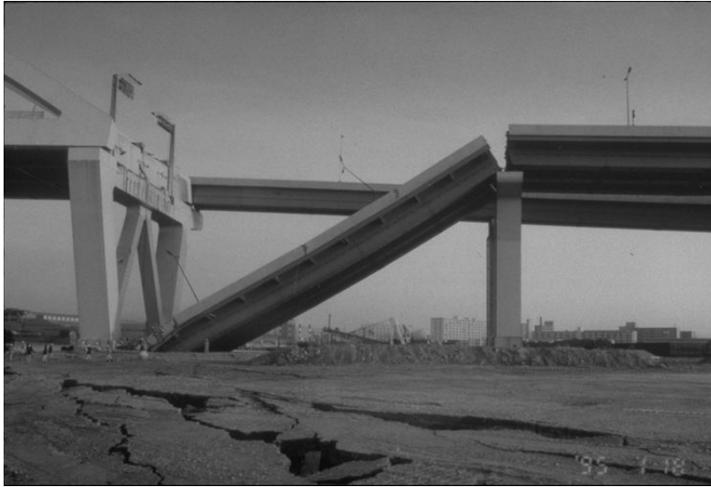
Figure 3.5. Nishinomiya Bridge following 1995 Hyogo-ken Nambu earthquake.
