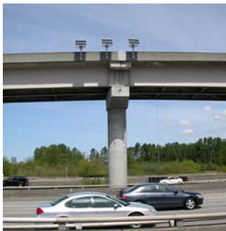
Automated data recorders on I-90 Mercer Slough near Bellevue (Source: WSDOT Bridge Office)
