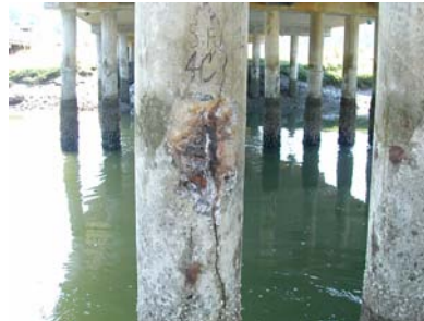
U.S. 101 Mudd Bay Bridges, Eld Inlet: Deteriorated concrete columns to be fitted with fiberglass jackets (Source: WSDOT Bridge Office)
