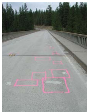
This repair and overlay project for the SR 231 Spokane River Bridge will remove the delaminated concrete and add a new modified concrete overlay. (Source: WSDOT Bridge Office)
