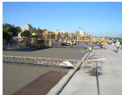
Workers on the I-90 Viaduct in Spokane replace the existing latex modified concrete overlay with a fly-ash modified concrete overlay. (Source: WSDOT Bridge Office)
