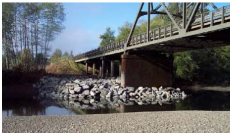
Rip rap placed around piers on the U.S. 101 Humptulips River Bridge (Source: WSDOT Bridge Office)
