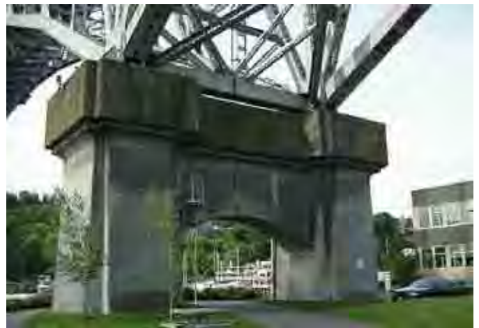
WSDOT is currently testing the effectiveness of using carbon fiber to help reinforce columns on the SR 99 Aurora Avenue Bridge.
