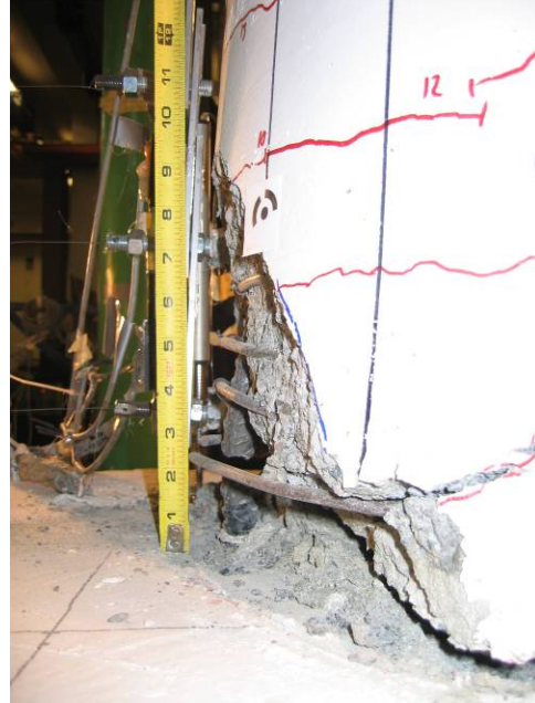
Figure 4-16. LB6-PT: Bar V00 fractured, Cycle 33 (6.75%).
