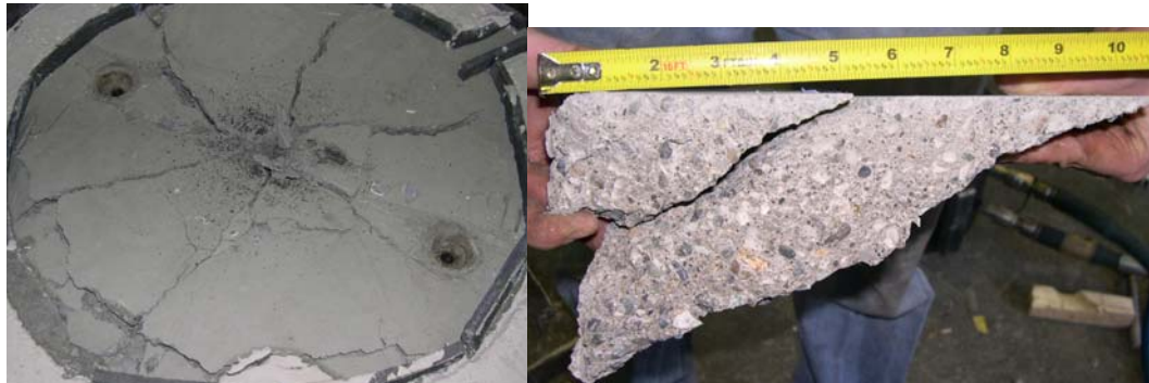
Figure 4.15: Concrete damage: 08C08
