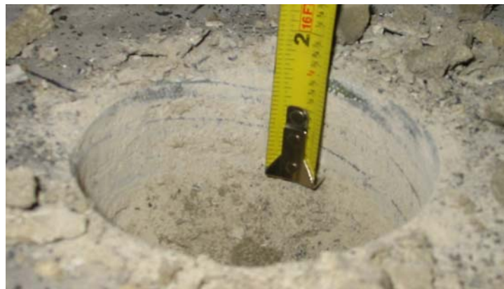
Figure 4.16: Grout damage: 08N08
