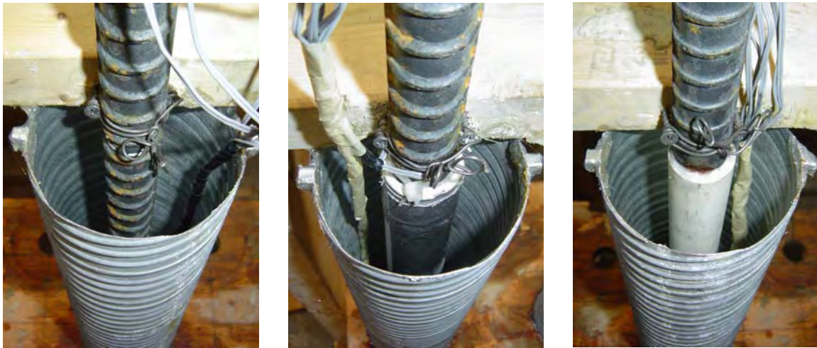
Figure D-2: Anchorage conditions in each specimen - AD8-FB (left), AD8-D1 (center), and AD8-D2 (right)
