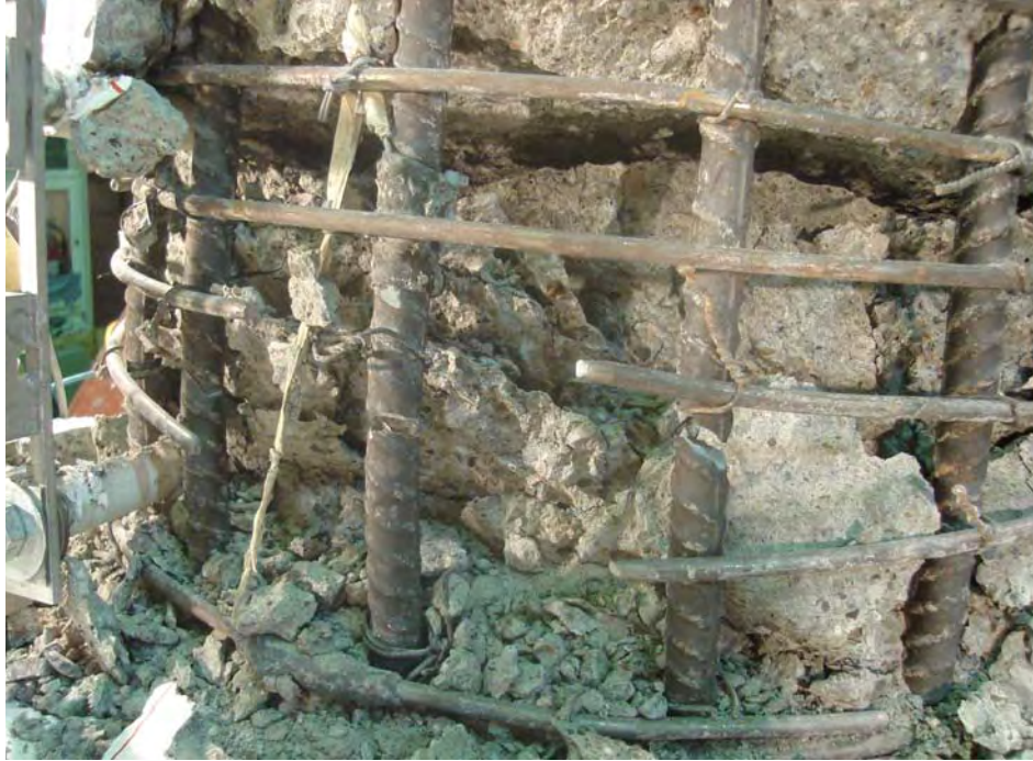
Figure 4-11: Bars 1, 2, and 16 fractured in Specimen DB5-RE at Cycle 36 (8.83%/-8.44%)
