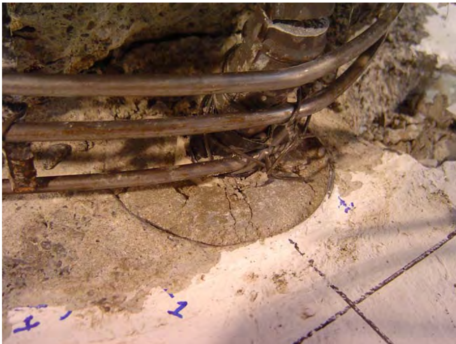
Figure 4-58: Specimen LB8-D2 with no spalling in the cap-beam; radial cracks in the grout at the end of testing
