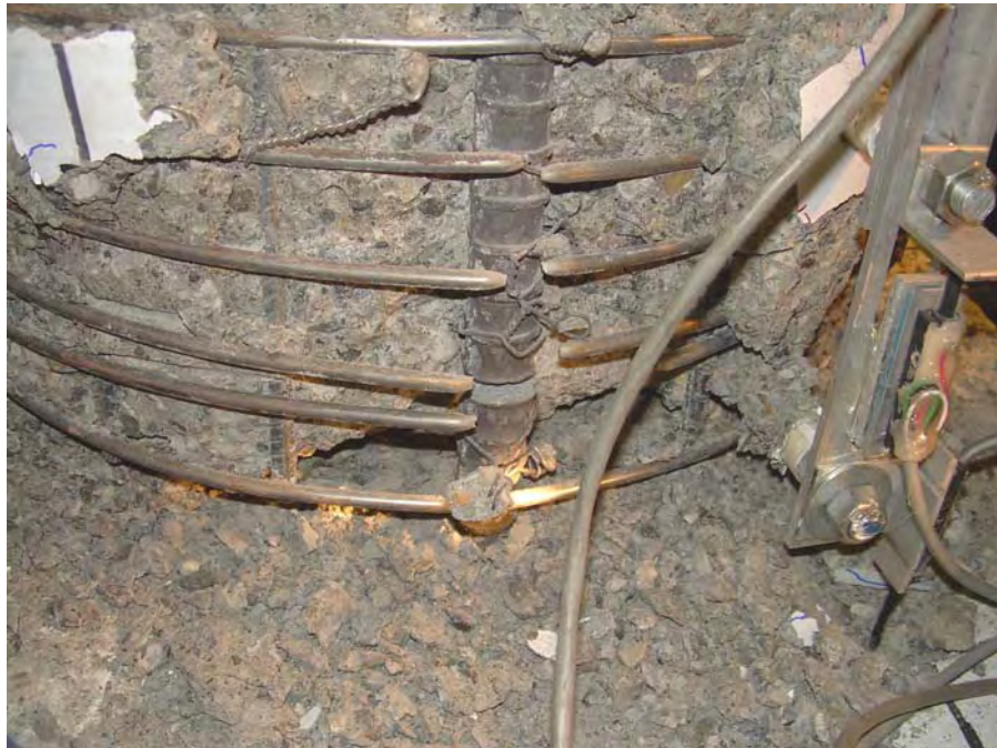
Figure 4-40: Bar 4 fractured in Specimen LB8-D1 during Cycle 34 (7.20%/-7.06%)
