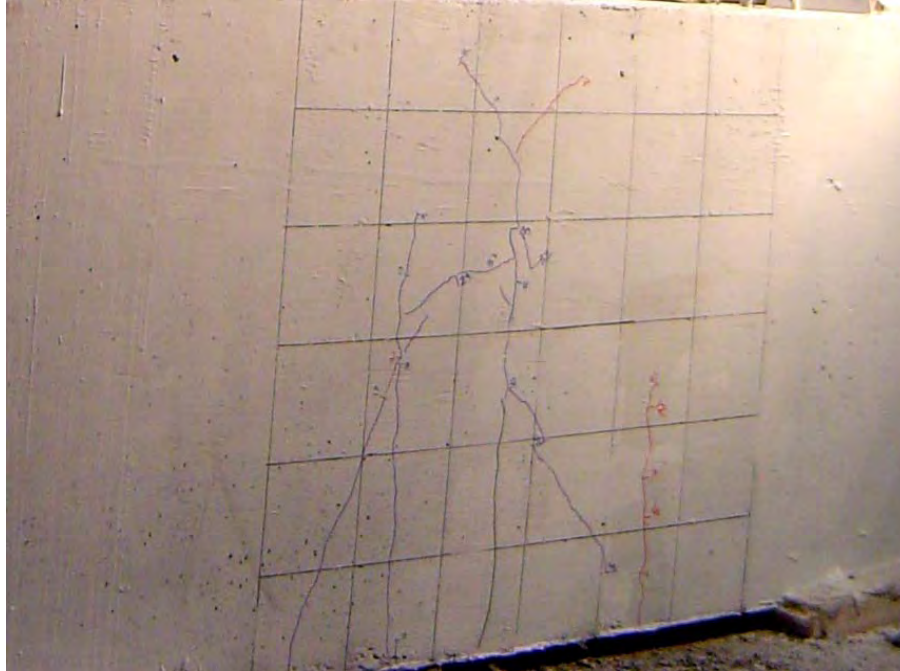
Figure 4-57: Damage to the cap-beam in Specimen LB-D2 after Cycle 34 (7.41%/-7.17%)
