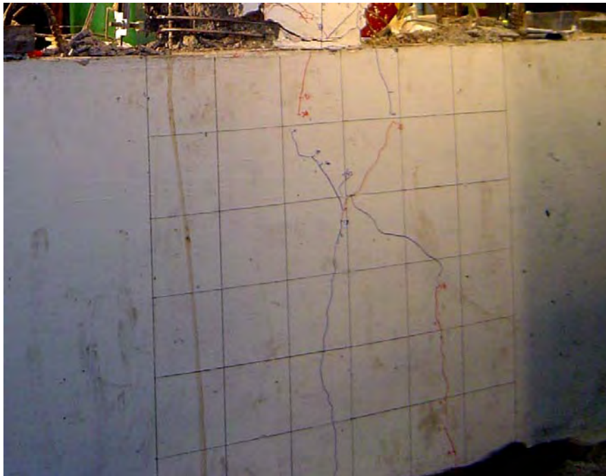
Figure 4-27: Cracking in the cap-beam in Specimen LB8-FB after Cycle 34 (6.81%/-6.40%)
