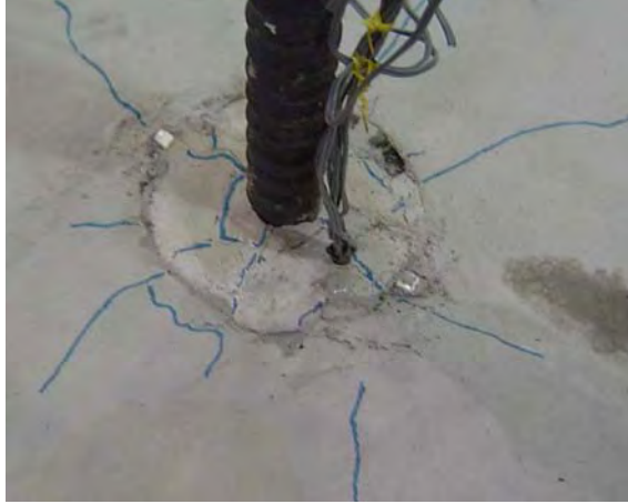
Figure D-10: Surface damage to Specimen AD8-FB
