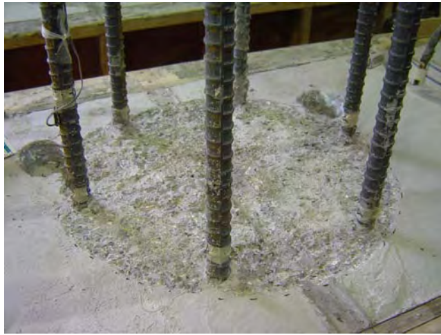
Figure B-32: Roughened surface of cap-beam under grout pad
