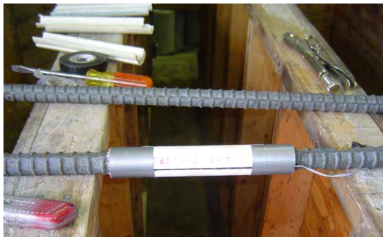
Figure B-20: Debonding of a #8 bar using Method 1
