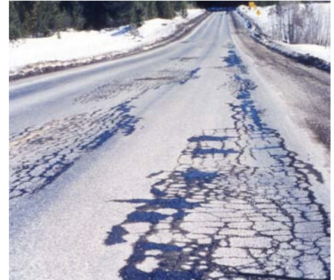
Photo 1. Example of the extent of damage caused by freezing and thawing on SR 20.
