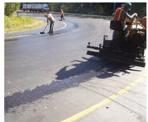
Brooming a sealer along the lane edge during surface preparation prior to placing the prime shot application.
