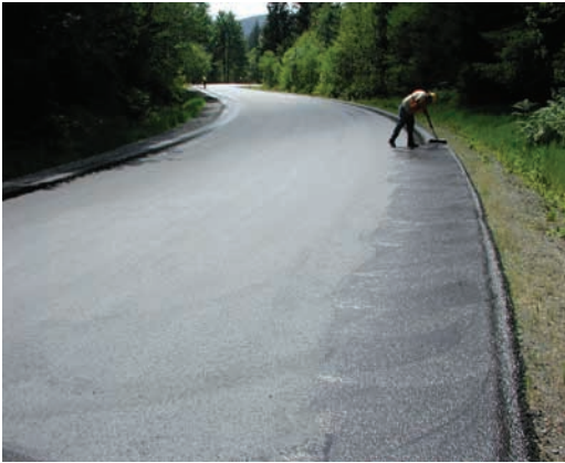
Preparation of shoulder surface by brooming along the shoulder edge after the prime shot has been applied.
