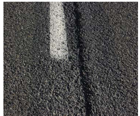
Image 1 - Joint in Washington with raveling and cracking present
