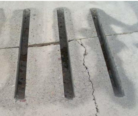
Photo 5. Slots cut to avoid longitudinal crack with accidental punchout through bottom of slot.
