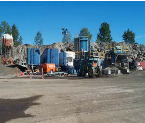
Photo 12. Slurry processing plant.
