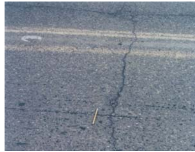
Photo 2. Low Temperature Cracking
