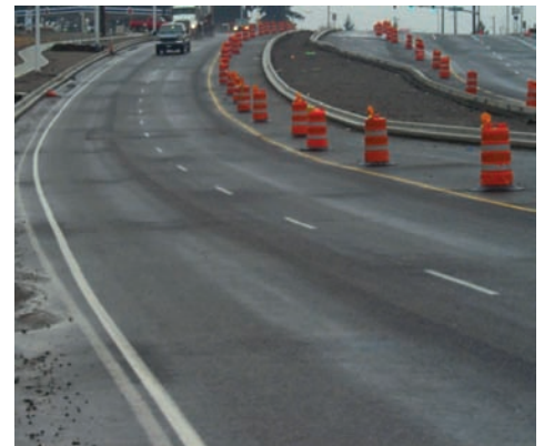
Image 1 - Segregated areas in pavement
