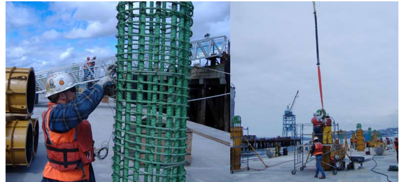
(left to right) A K-G worker ties rebar on a pontoon ZC/ZD column. April 7, 2008. K-G crews place concrete into a two-piece, steel form on pontoons ZC/ZD. April 16, 2008.
