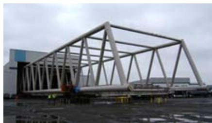
The Hood Canal Bridge's new west truss moves from the OIW facility, allowing crews to start assembly work of the new east truss. April 22, 2008.
