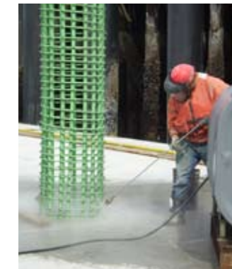
A K-G worker pressure washes concrete from column rebar on ZC/ZD in preparation for form placement at TPS. April 10, 2008.
