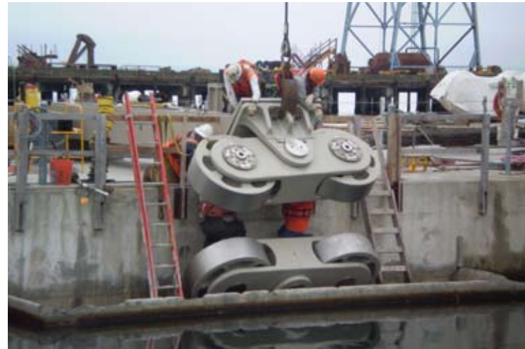
Crews at TPS install a roller guide into a draw span pontoon at TPS in Seattle. June 13, 2008.
