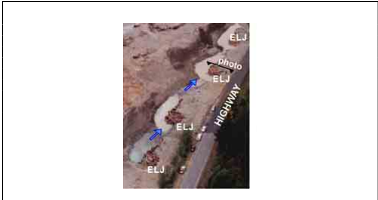
Figure E-16. Installation of ELJs flow deflectors in the Cispus River after a flood event that razed a poorly developed riparian buffer and damaged a portion of the highway.
