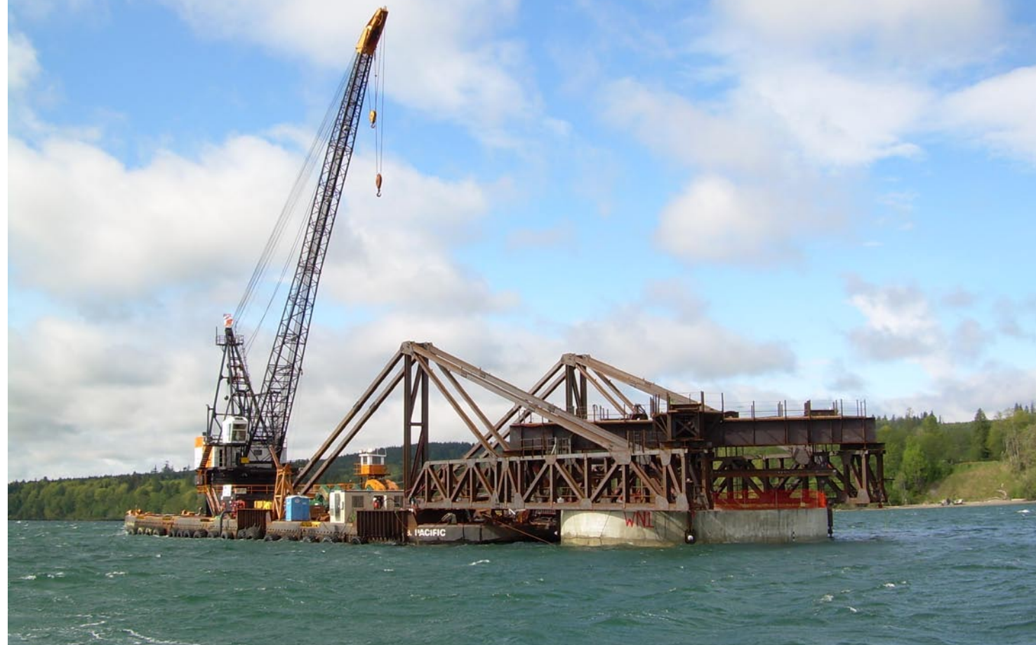
Crews complete anchor setting tests using a barge with a truss section that was specifically built for this operation, April 24, 2007.
