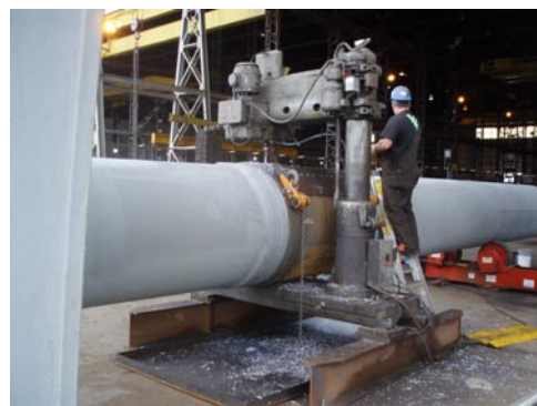
Crews drill holes for the floor beam connections to a bottom chord, September 20, 2007.
