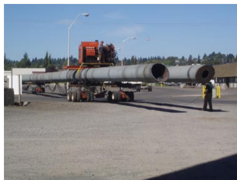
Two truss top chords are transported to a larger facility where assembly will occur, September 24, 2007.
