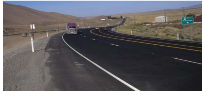
The newly constructed truck passing lane on SR 24 is designed to improve safety and accommodate freight mobility.
