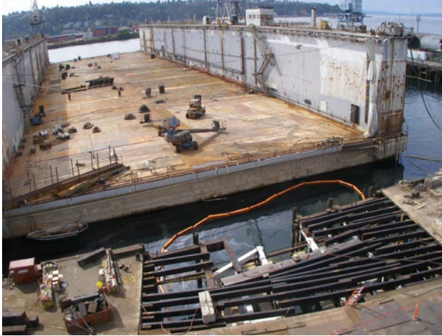
Dock for anchor construction at Todd Pacific Shipyards floats in place. August 22, 2006
