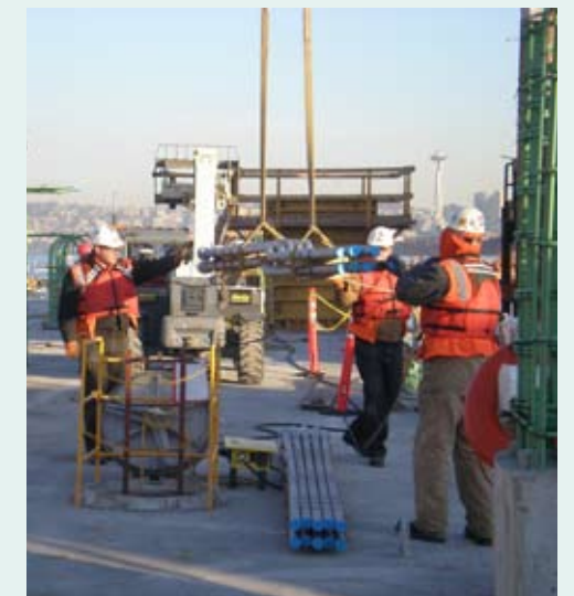
Kiewit-General crews help a crane guide pipe spools onto pontoon PB Jan. 25, 2008.
