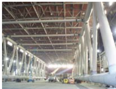
Transition spans fill an enormous building at Oregon Iron Works in Vancouver, Wash. Crews at the site are working to connect top struts on the bridge section, which measures approximately 280 feet long, 70 feet wide and 40 feet tall Jan. 15, 2008.
