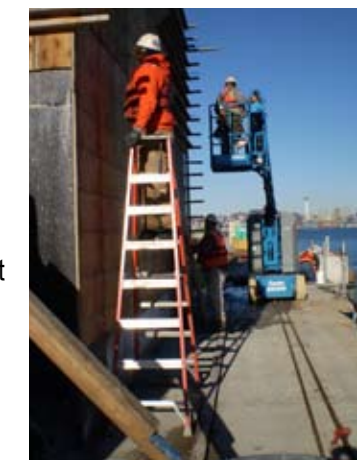
Crews strip the forms used on the electrical building on pontoon Q at Todd Shipyards in Seattle. Once completed, the building will serve as one of two electrical buildings on the draw span Jan. 21, 2008.
