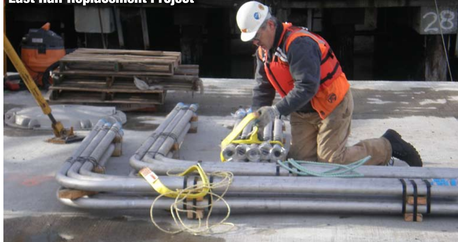
A worker prepares hydraulic piping so it can be installed in the cells of pontoon PB Jan. 9, 2008.
