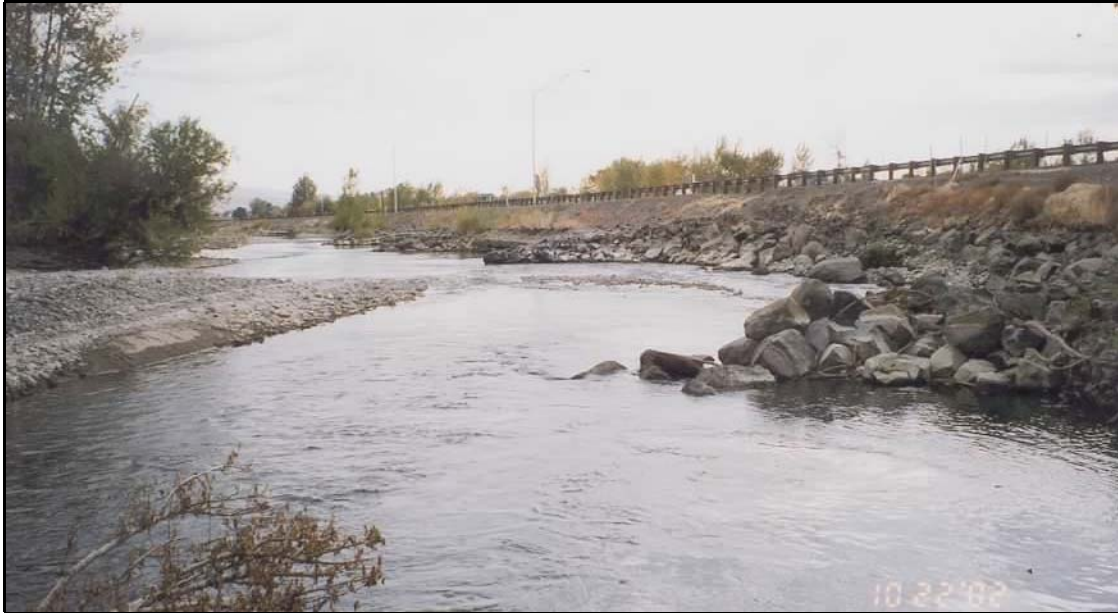
Figure 7: Photograph taken from Station 7800 looking downstream at recent efforts to protect the road prism of US 12. Note railing along edge of eastbound lane of US 12
