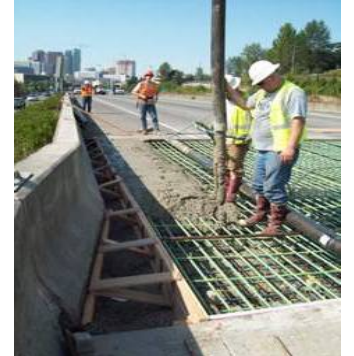
Crew Member Pouring Approach Slab on North End of NE 8th Street.
