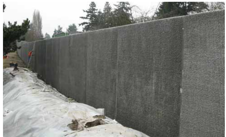
Crew member working on the highway side of Wall 2 near NE 92nd Street.
