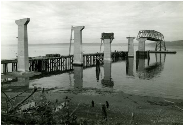
Crews construct columns and a transition span for the Hood Canal Bridge in 1958.
