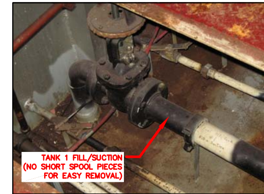
PHOTO 10-C FO STORAGE TANK 1 FILL/SUCTION
