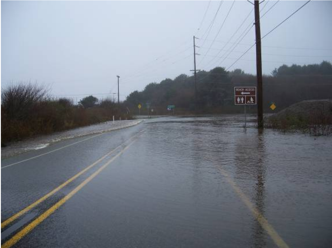
Figure 4. Flooding on SR 109 north of the Moclips River bridge in March 2007.
