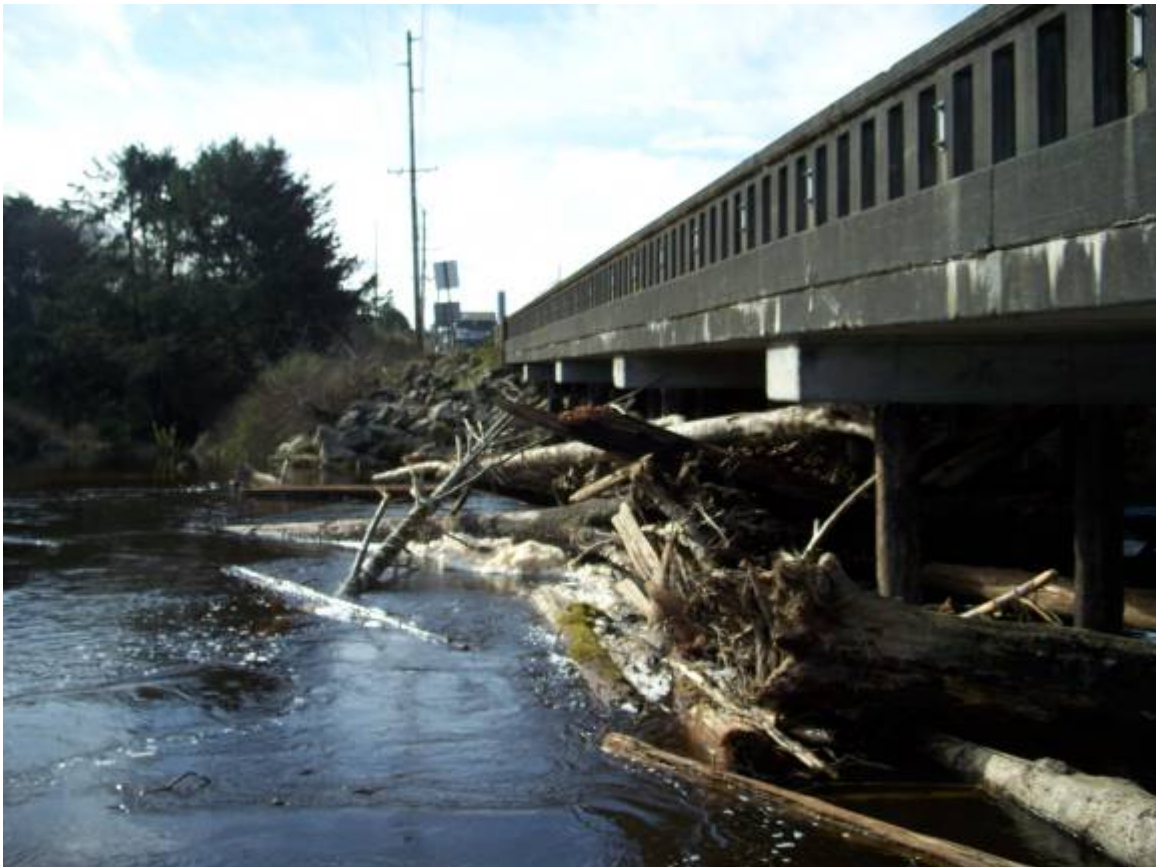
Figure 3. Log jam accumulation on the underside of the Moclips River bridge structure (looking south, March 2007).
