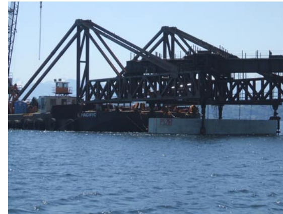
The Derrick Barge Pacific lowers the tenth anchor to the bottom of Hood Canal, May 30, 2007.
