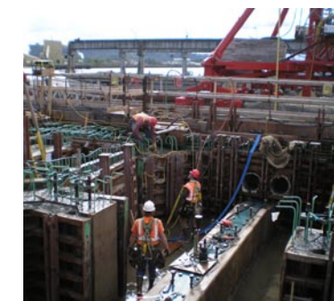
Crews strip the upper half panels of the anchor gallery on pontoon NA. May 03, 2007.
