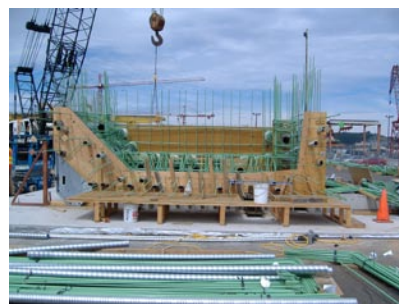
Ironworkers tie rebar for a cycle three pontoon pre-cast exterior wall section, May 30, 2007.
