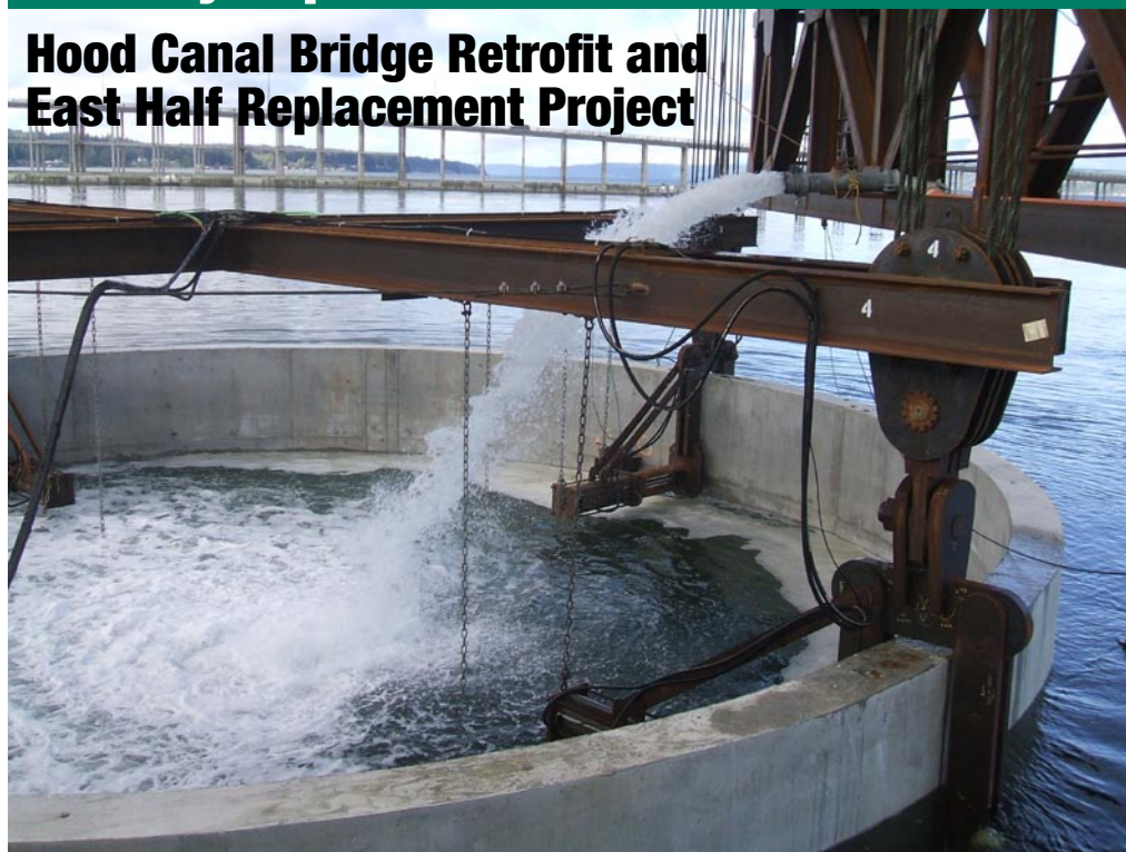
Sea water cascades in to the middle of the anchor before it is lowered to the bottom of Hood Canal, May 3, 2007.
