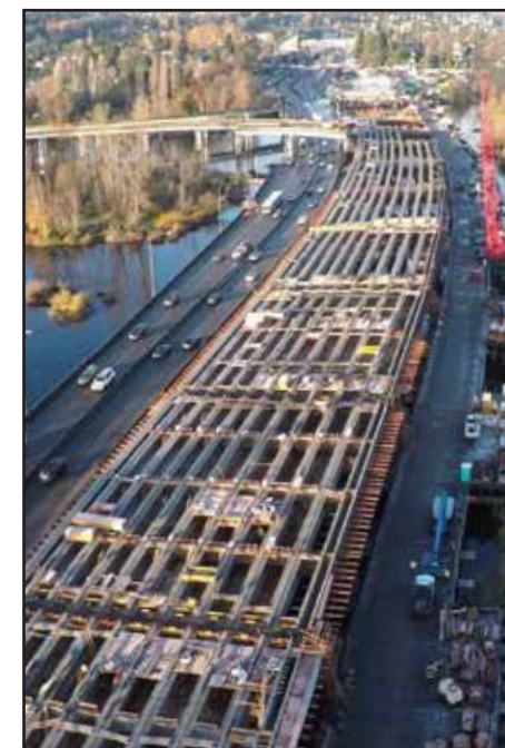
December 2016 view, looking west, of the West Approach Bridge North under construction.
