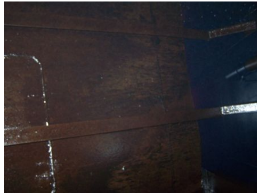
Storage Tank Bottom Above Suction Line (S013.jpg)
