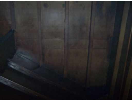
Storage Tank Bulkhead, #2 End Frame-6, Bottom (S004.jpg)
