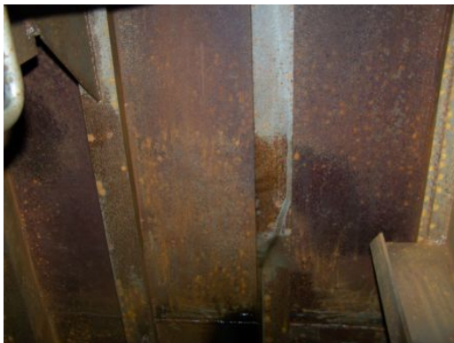
Day Tank Overhead (D001.jpg)
