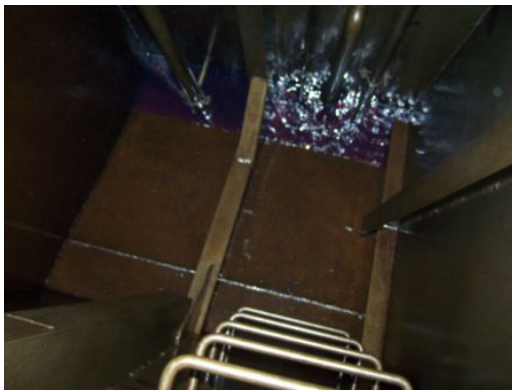
Day Tank Bottom (D006.jpg)
