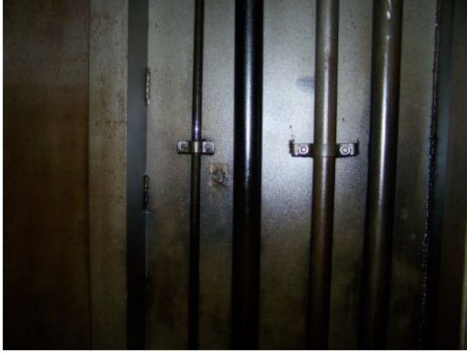
Day Tank Bulkhead, Inboard (D003.jpg)
