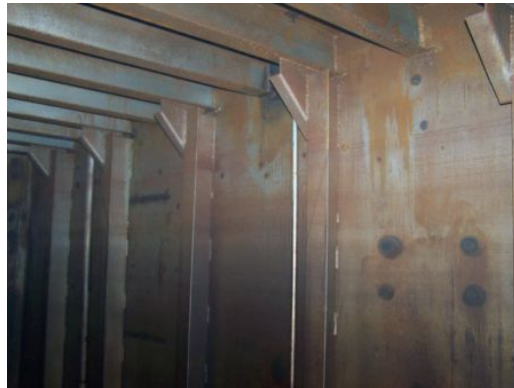
Storage Tank, Inboard, Top (S005.jpg)
