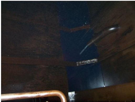
Storage Tank Bottom Above Suction Line (S012.jpg)
