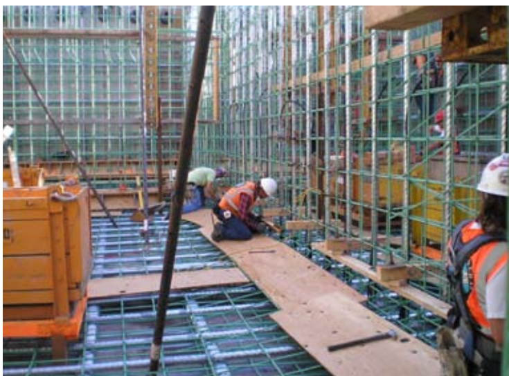
Crews from Kiewit-General install wall forms into pontoon X at CTC in Tacoma. Aug. 27, 2007
