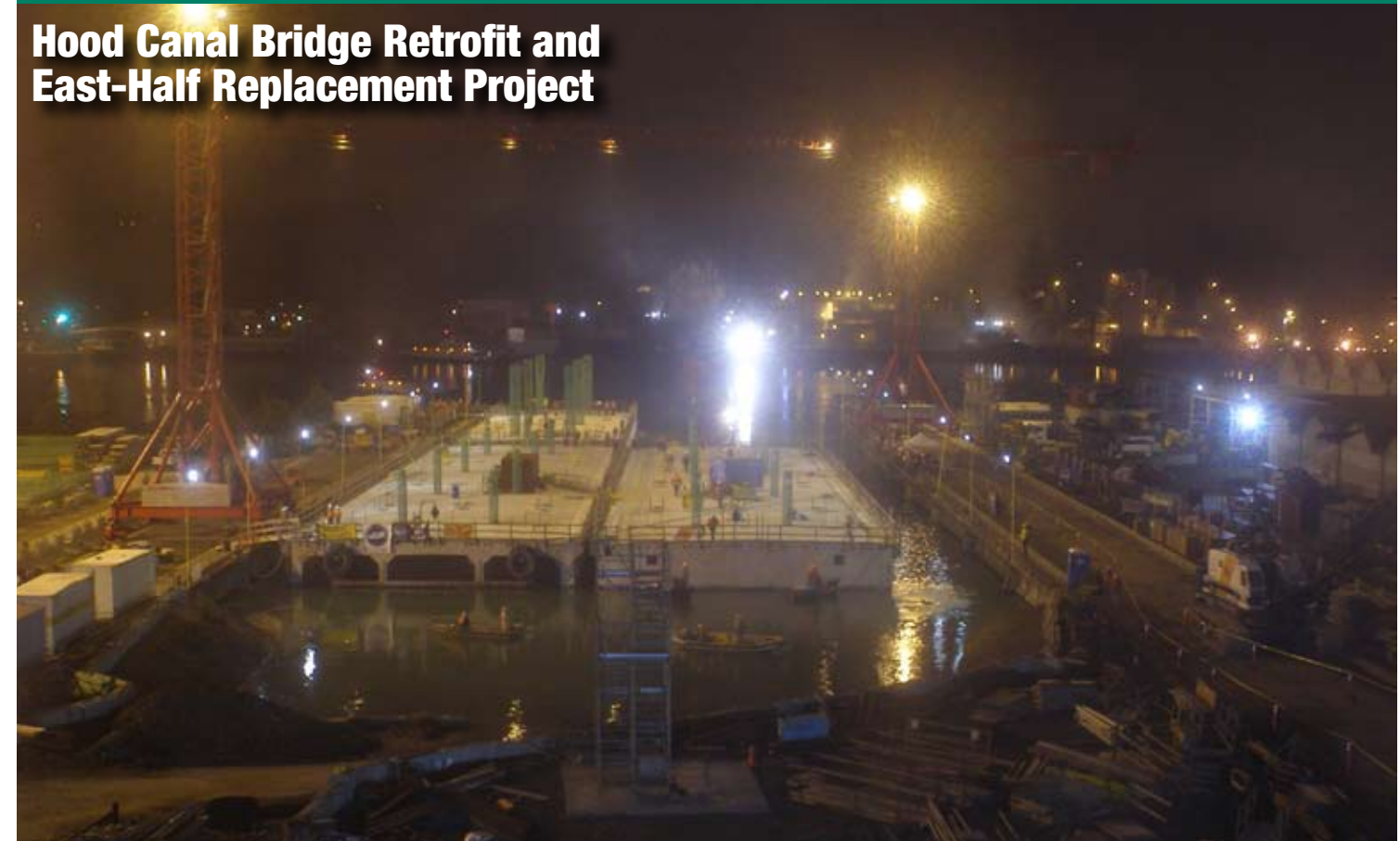
With pontoon X clear of the graving dock, crews from WSDOT, Kiewit-General and Foss Tugboats prepare pontoon ZD for float out at Concrete Technology Corporation in Tacoma. Feb. 21, 2008.
