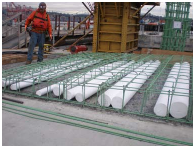
A Kiewit-General crewmember installs Styrofoam fillers in the lower ramp of pontoon PB at Todd Pacific Shipyards in Seattle. Feb. 12, 2008.
