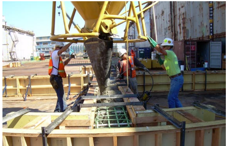
Laborers pour concrete for two-foot tall lower spokes and anchor footing section, September 12, 2006.
