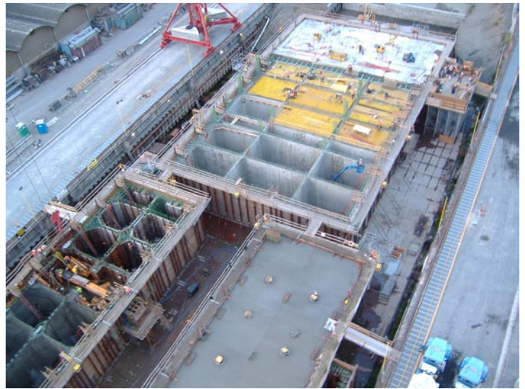
This is an aerial photo showing work completed on the cycle one pontoons. Wall pours on Pontoon Q (top) are complete, deck pours on pontoon PA (lower right) are complete and walls are ready to be poured on pontoon PB (lower left), August 8, 2006.
