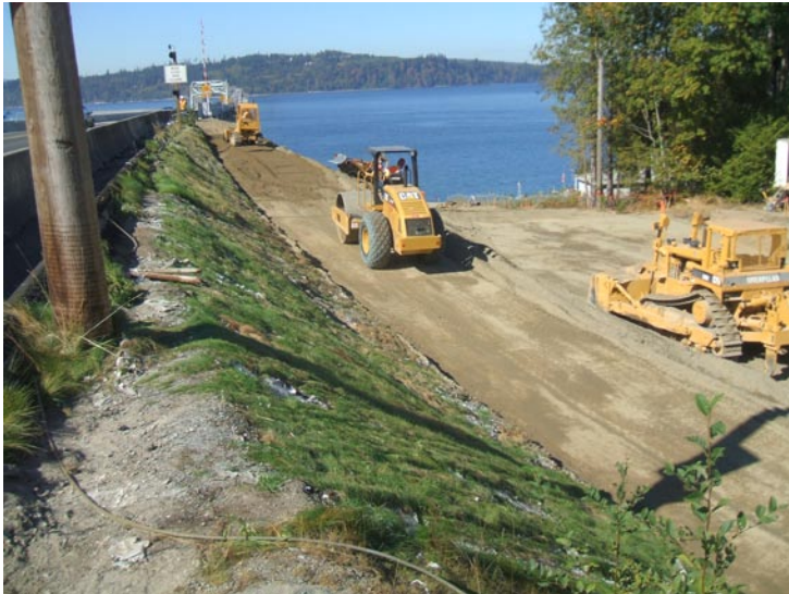
Crews work near the east approach span to restore the bank, September 29, 2006.
