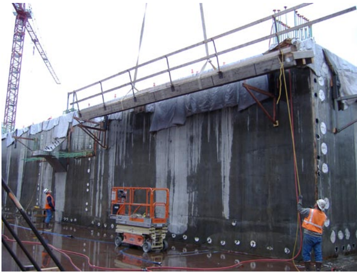
Tower crane operator lowers work decks to the side of pontoon PA for post tensioning operations, August 17, 2006.
