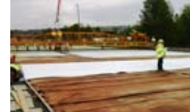
Crews place a tarp over new concrete for the Oakesdale bridge deck.
