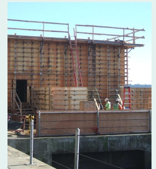
Carpenters complete the diesel tank wall enclosure forms on the west-half electrical building, October 23, 2007.
