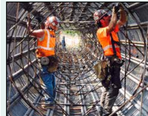
Crews hand tie rebar cages that will strengthen concrete columns for the West Approach Bridge North.
