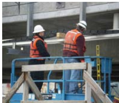
K-G crews install the cable tray on the draw span pontoons. Feb. 23, 2009.
