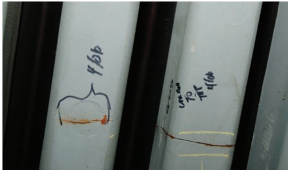
The joints are continuing to crack and deteriorate, requiring constant maintenance.
