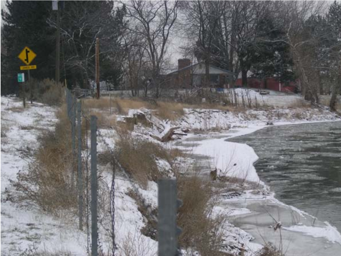
Figure 1. Left bank erosion on the Yakima River at SR 224/Van Giesen Road.
