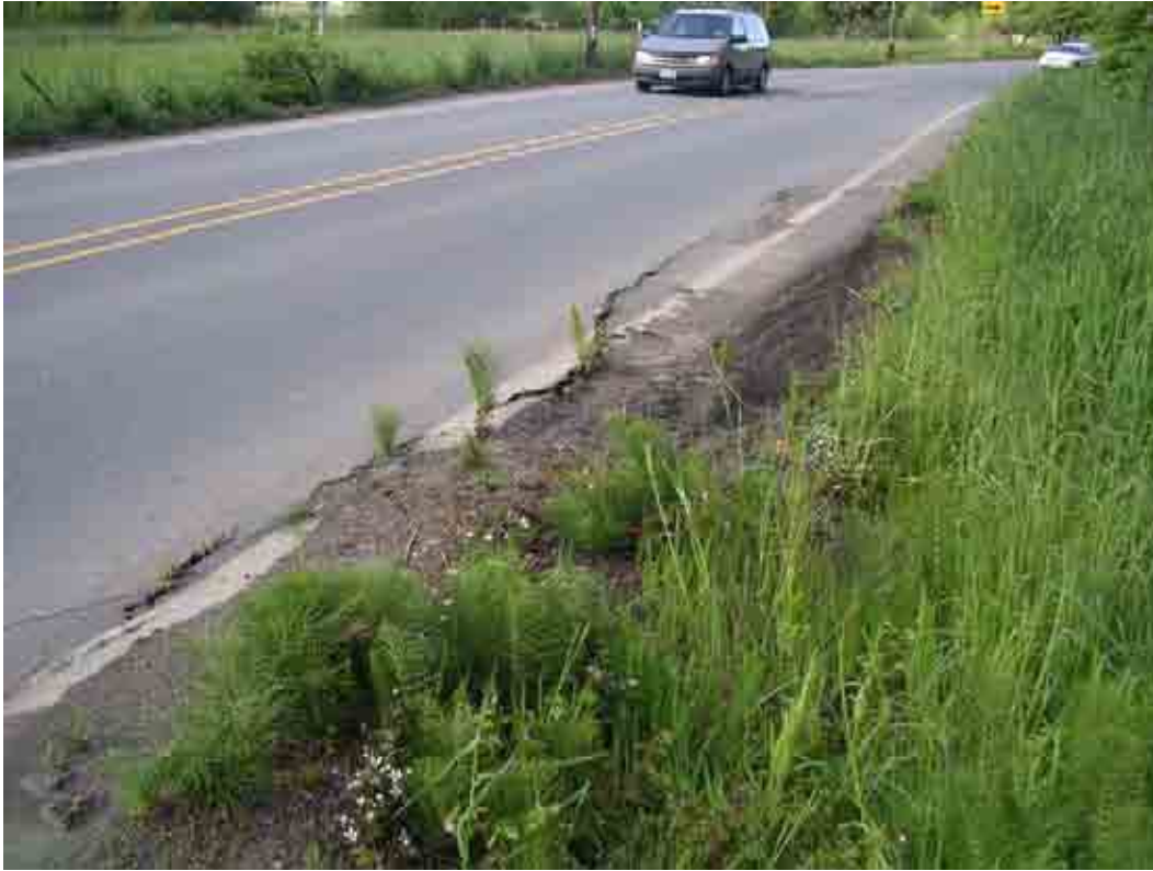
Photo A-31. Pysht River Site ID P-3 (May 11, 2005). Detailed view of cracked pavement. Area where road cracks are exhibited is approximately 55 feet in length. End of cracking downstream is coincident with the start of rip rap (41 feet downstream of 30MPH sign). (Photo 2500)
