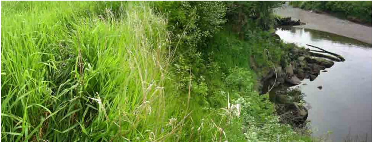
Photo A-9. Hoko River Site ID H-1 (May 12, 2005). Looking downstream at undercutting of gravel sand toe of bank, apex of meander at MP 11.42. (Photo Pan 2571-2574)
