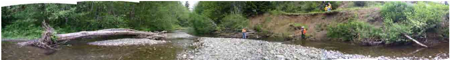
Photo A-17. Clallam River Site ID C-2 (May 11, 2005). Looking at right bank erosion – 220 feet of erosion. (Photo Pan 2395-2401)
