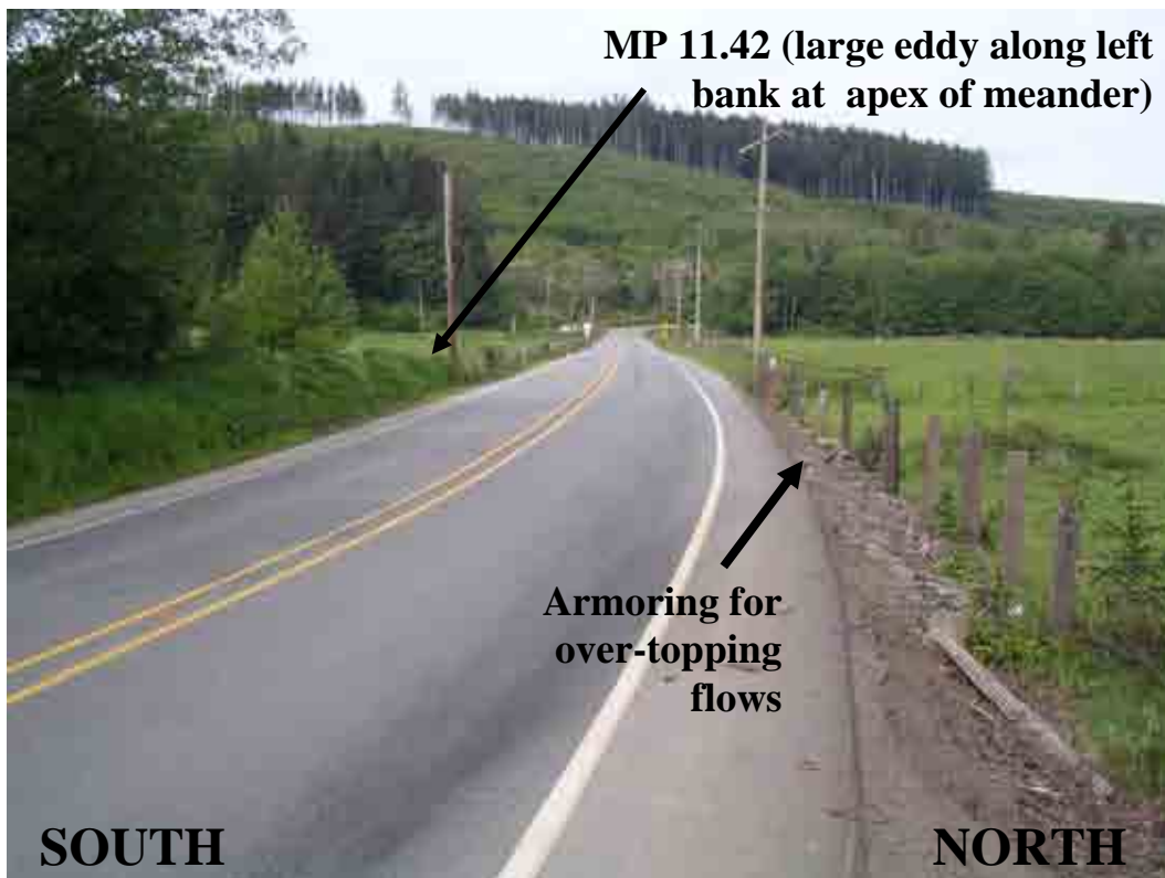
Photo A-10. Hoko River Site ID H-1 (May 12, 2005). Looking west at upstream end of H-1, MP 11.42. Road is raised about 4 feet above floodplain and still susceptible to overtopping flows (note armoring along downstream or north (right) side of road. (Photo 2575)
