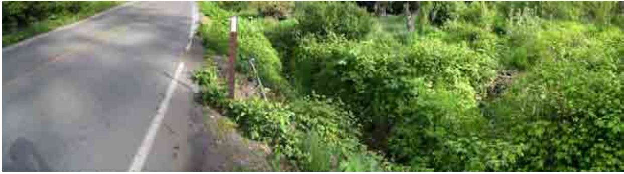
Photo A-12. Hoko River Site ID H-2 (May 12, 2005). Looking west along SR112 and upstream of culvert. Tension cracks in pavement are visible for 25 feet along the right shoulder. (Photo Pan 2530-2532)
