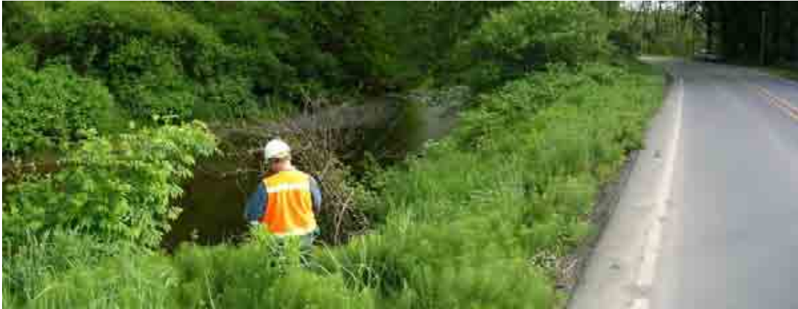
Photo A-29. Pysht River Site ID P-03 (May 11, 2005). Looking upstream . Bank height is approximately 15 feet. Top of bank is 9 feet from the edge of the pavement. Bank erosion – 40 feet. Limited riparian vegetation. (Photo Pan 2497-2498)
