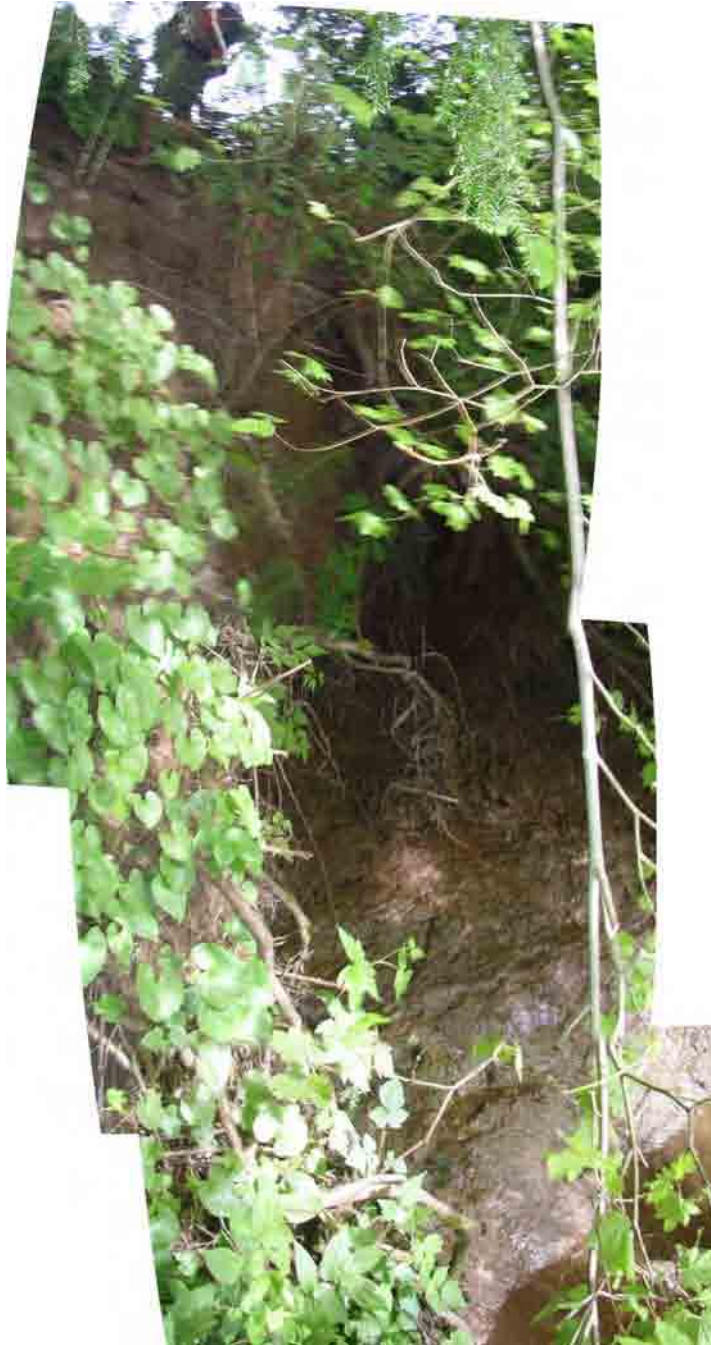
Photo A-69. Pysht River Site ID P-7 Bank erosion. Near MP 28 (108 yards downstream) right bank is 18 feet high (sand). Photo above illustrates bank calving. (Photo Pan 2424-2426)
