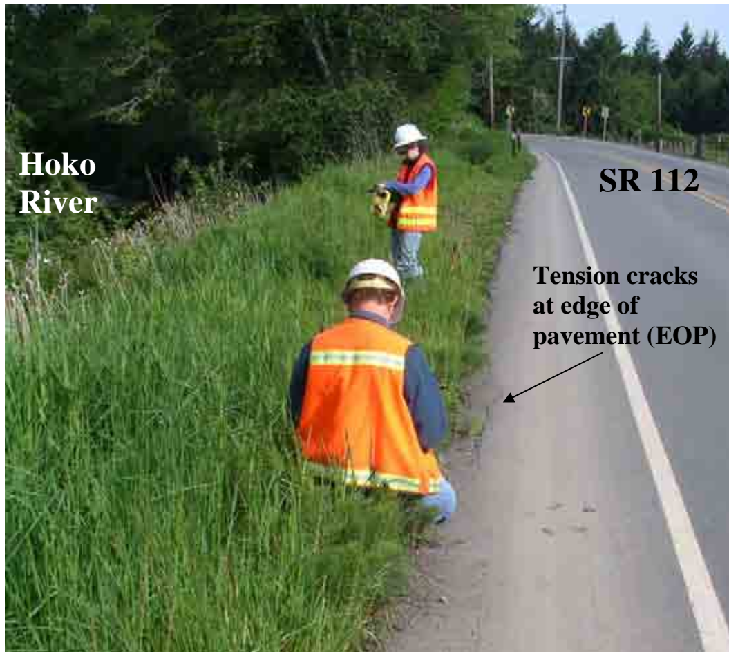
Photo A-1. Hoko River Site ID H-1. (May 12, 2005). Looking west at tension cracks in SR 112 pavement due to bank slumping along Hoko River. Cracks are approximately one foot from the edge of pavement extending 25 feet along the road at MP 11.5. (Photo 2537)
