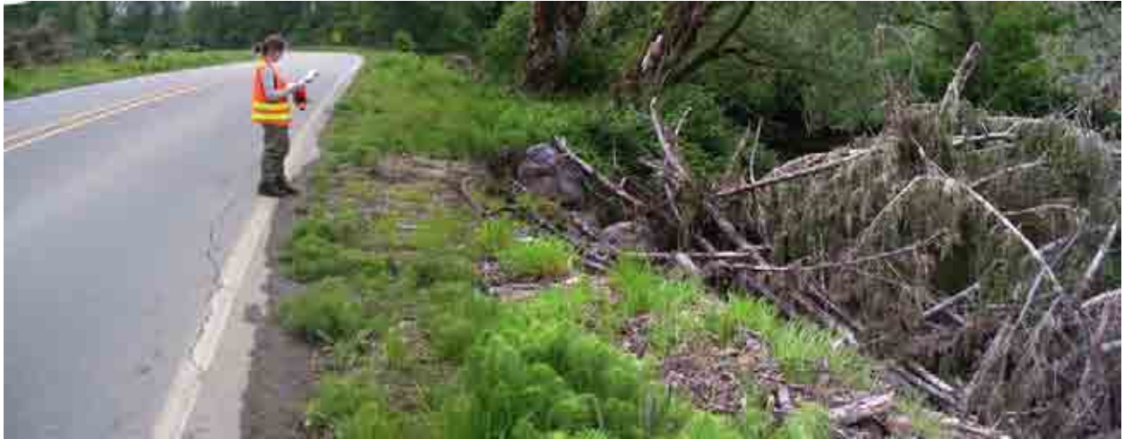
Photo A-59. Pysht River Site ID P-5 (May 10, 2005) 48 feet of cracked pavement just downstream of P24 (Photo Pan 2313-2314)
