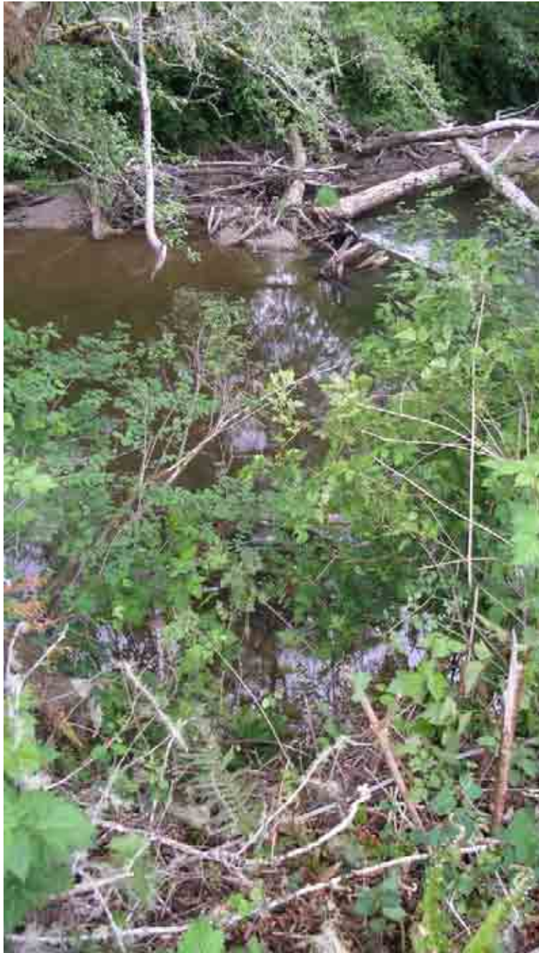
Photo A-66. Pysht River Site ID P-5 (May 10, 2005). Vertical panoramic of top edge of right bank with steel cable (to log downstream along recent repair site) immediately downstream of alder clumps leaning into river. Upstream of alder clump is rock rip rap. (Photo Pan 2330-2332.)
