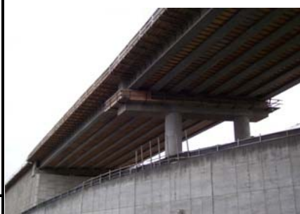
New southbound bridge over I-90 opened to traffic the night of December 15th
