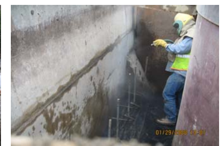
Crew member sand blasts in preparation for final lift of blister pour at Pier 6, I-90.
