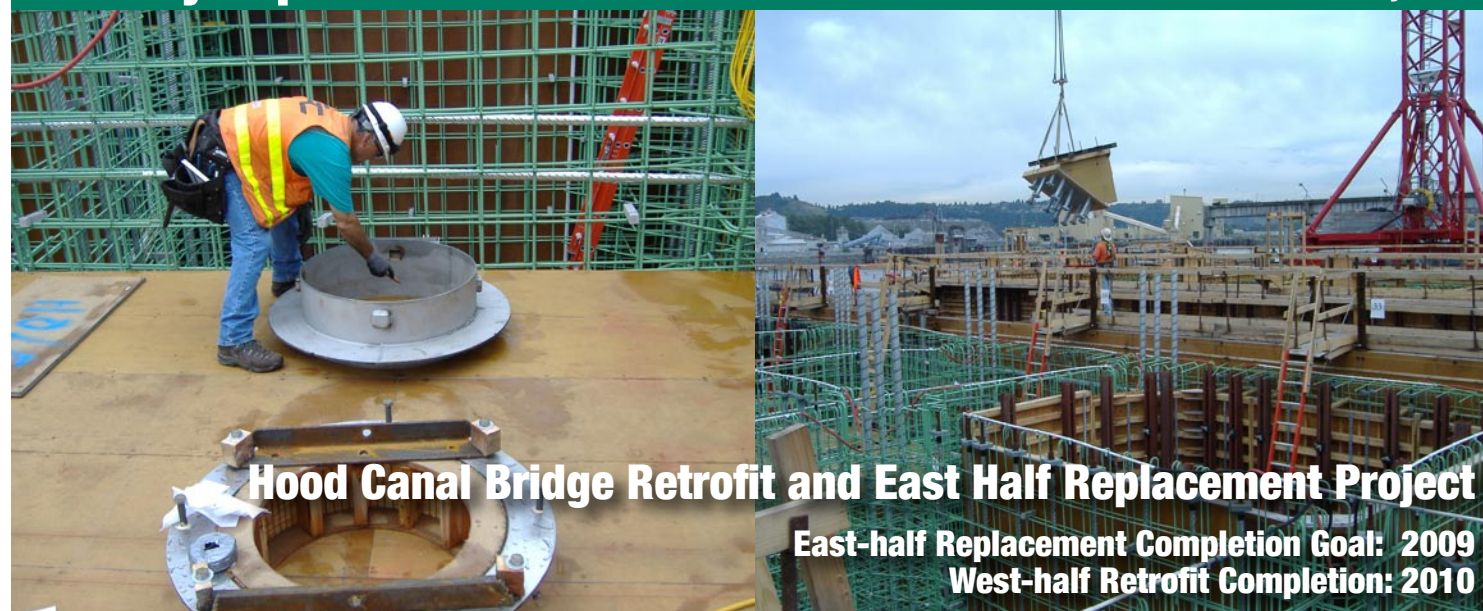
Worker installs interior hatch cover components in one of the pontoon PA anchor galleries. May 31, 2006
