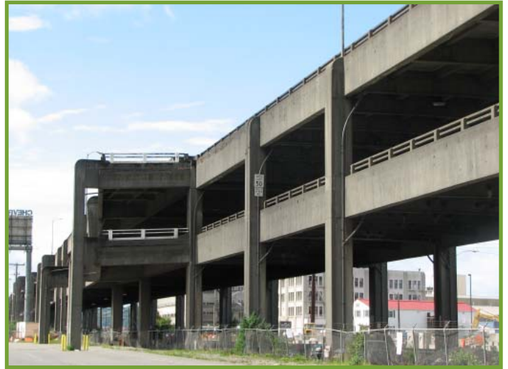
The viaduct's south end is vulnerable because it sits in unstable soil that could liquefy in an earthquake.
