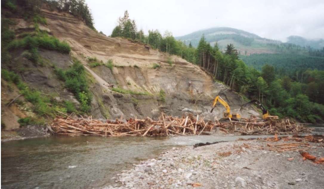
Figure I-5: LWD revetment constructed as part of the South Fork Nooksack, Larson’s Bridge Project, approximately RM 20.
