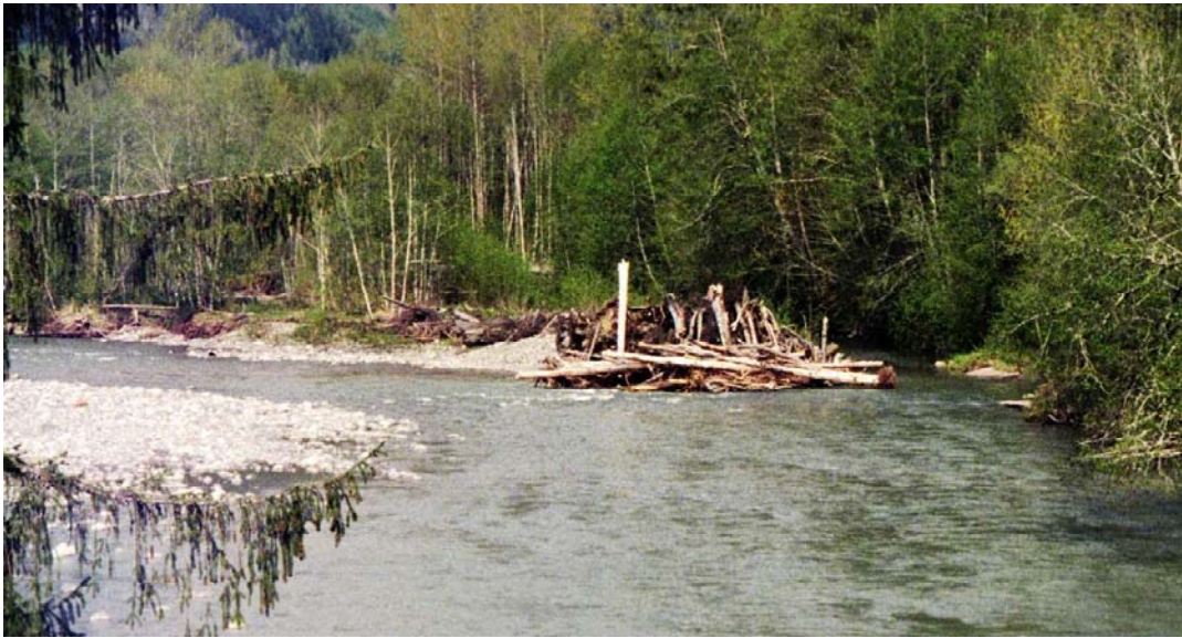
Figure I-9: ELJ constructed as part of the South Fork Nooksack, Larson’s Bridge Project.
