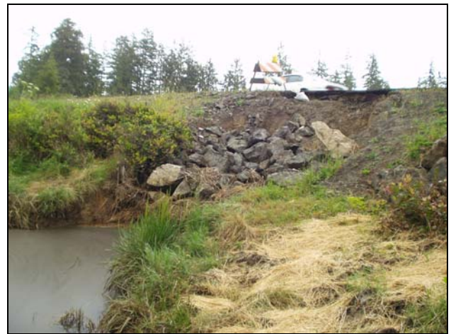
Figure 2. 2003 photo of collapsing shoulder at the culvert inlet.
