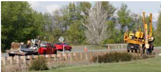
Construction begins on the Yakima River to West Ellensburg paving project, funded by Recovery Act dollars.
