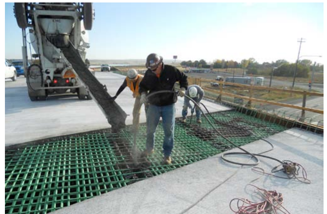
Pouring concrete for the new bridge crossing over US 12 at Humorist Road. November 2011
