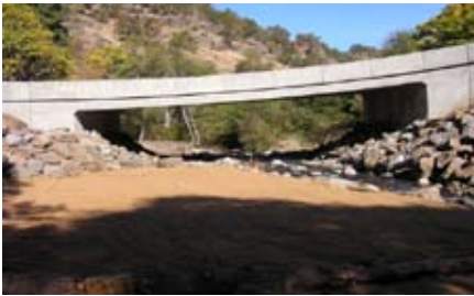
AFTER: A new 60 foot bridge restored fish passage for coho salmon, steelhead, bull and resident cutthroat trout.
