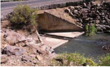
BEFORE: SR 142 near Goldendale and Bowman Creek. A 9 foot box culvert was a velocity barrier during high flows and prevented fish passage.
